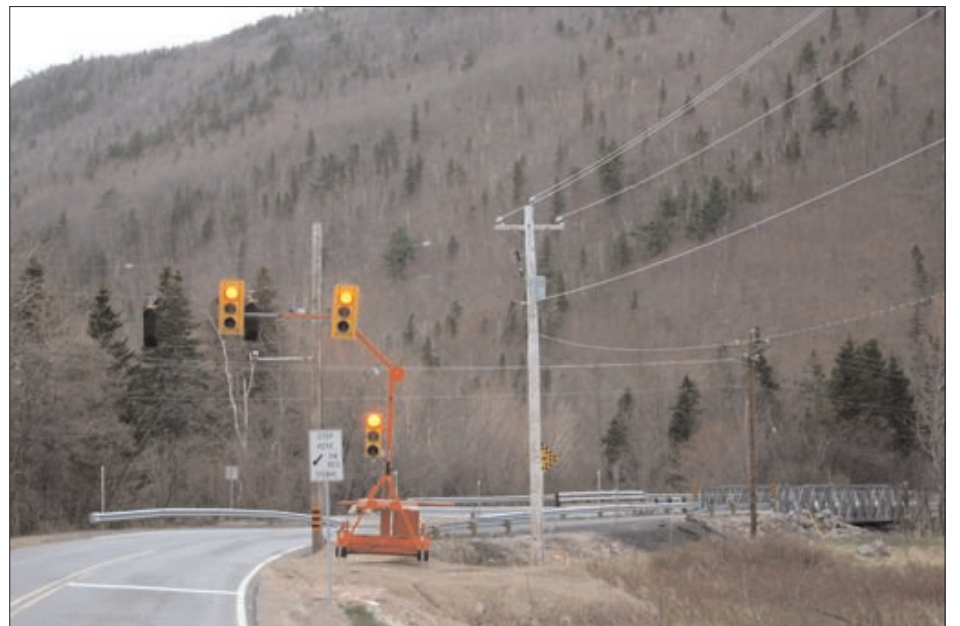
Waiting for the lights at Corson Bridge in Ingonish Ferry will frustrate drivers for a few more months. Engineer Kim MacDonald at the Department of Transportation says the new bridge is being designed and built this spring and summer with installation expected in the late fall.
